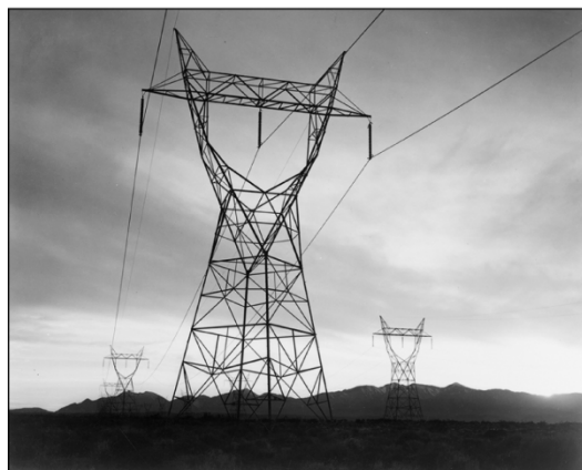
Figure 4: High-voltage transmission lines
